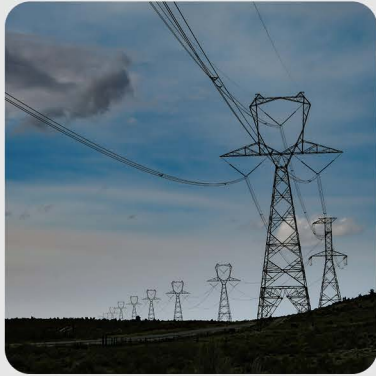
Peak off-peak electricity prices Store electricity when electricity prices are low and use it during peak electricity prices to reduce energy costs.
